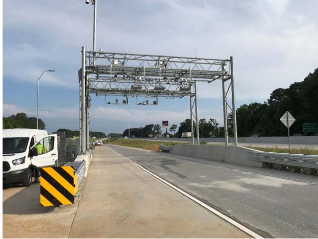
Figure 3 Example of Northwest Corridor Express Lane toll gantry at Big Shanty Road
